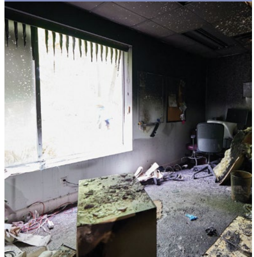
Some of the firebombing damage at the CompassCare in Buffalo, NY on June 7, 2022. The arsonists graffitied "Jane was here" on the building, referring to the group Jane's Revenge which had been promoting a "Night of Rage" ahead of the potential reversal of Roe v. Wade .
